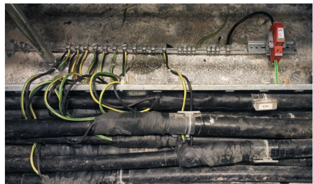
Indirect earthing of armouring and shields of cables to the technical building, to avoid disturbance by interfering voltage
