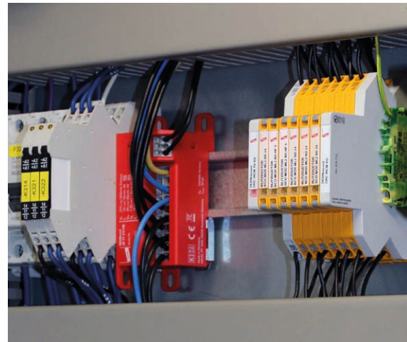
Figure 17 Example use of the BLITZDUCTORconnect in the technical building equipment
